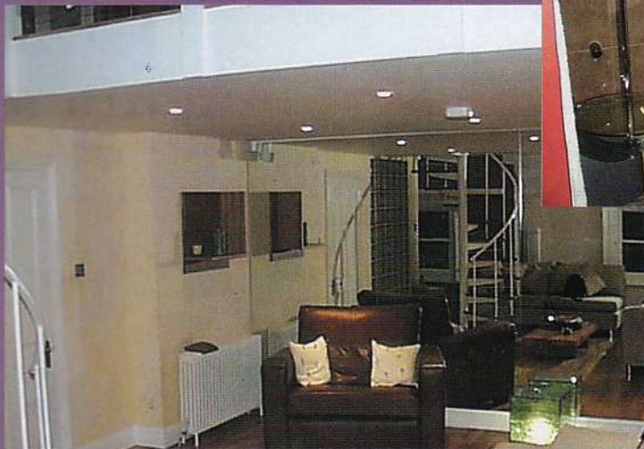
Clockwise, from top left: The work starts, laying the dining room floor, the sauna-steam room in the main bedroom, a spiral staircase dominates the main living room, the guest room is one of two which has luxurious carpet
